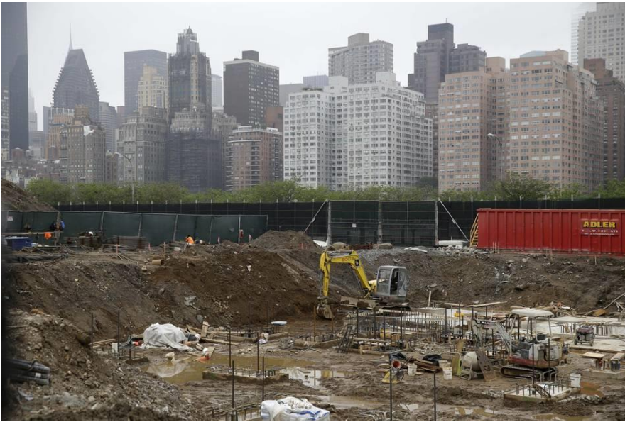
Construction on the Cornell Tech campus on Roosevelt Island in June. PHOTO: SETH WENIG/ASSOCIATED PRESS
